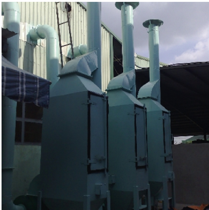
Factory dust extraction system
