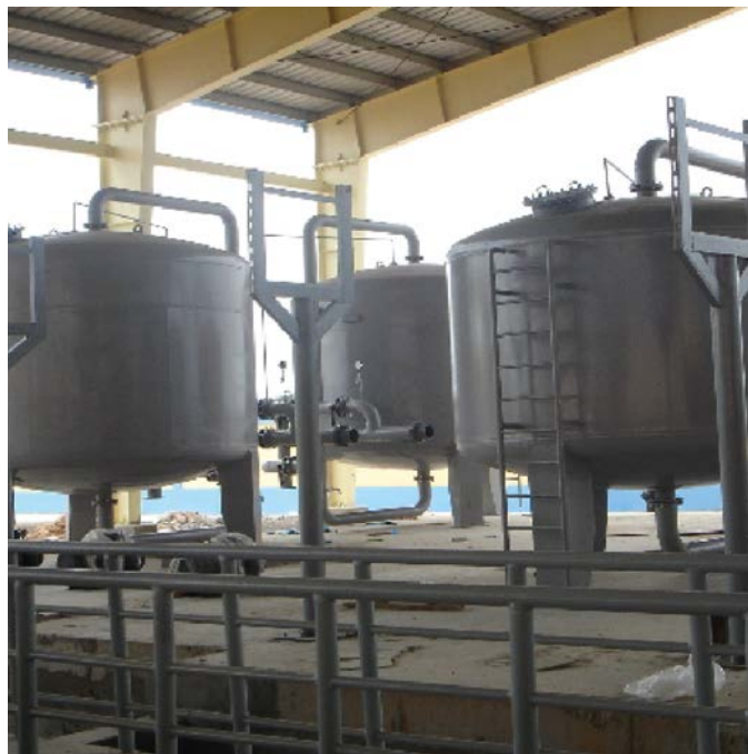
Industrial wastewater treatment system
