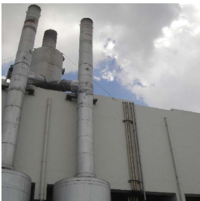
Generator smoke treatment system
