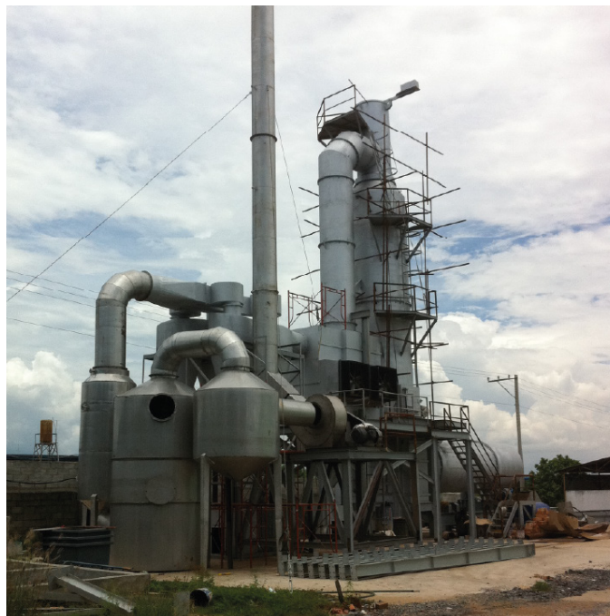
Hazardous waste incineration station
