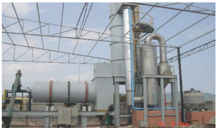
ENVIRONMENTAL TREATMENT SYSTEM
