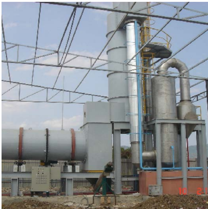
Industrial solid waste incineration system
